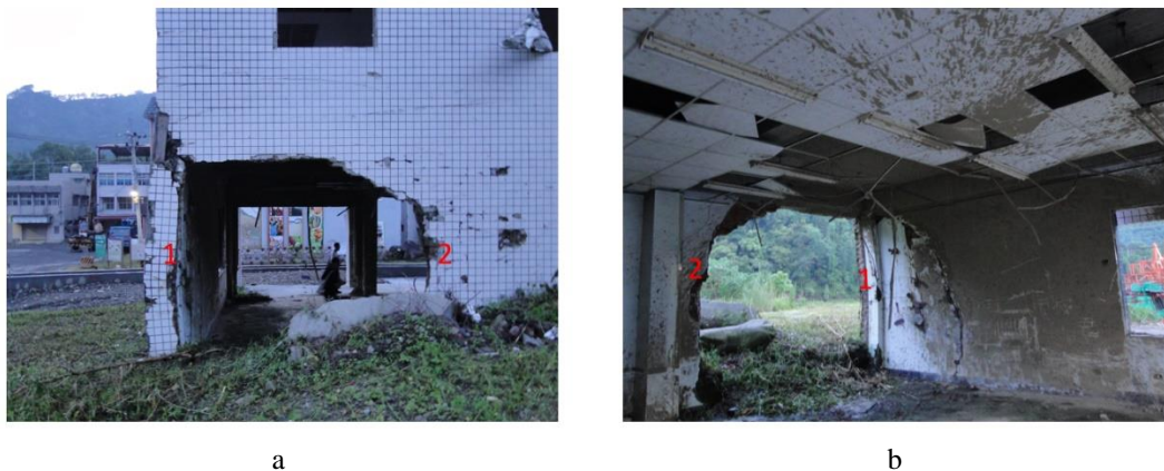
Fig. 1. The debris-flow front caused badly damage to a building in Nansula Village during Typhoon Morakot on 08/09/2009 (picture taken on 06/06/2013): a – the debris-flow front with boulders caused severe damage to the building during Typhoon Morakot (08/09/2009); b – the mud splatters remained on the inside ceiling of the damaged building
