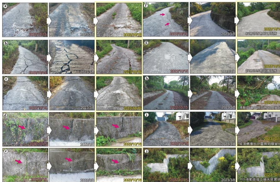
Fig. 7. Comparative photos of changes in surface fissures
